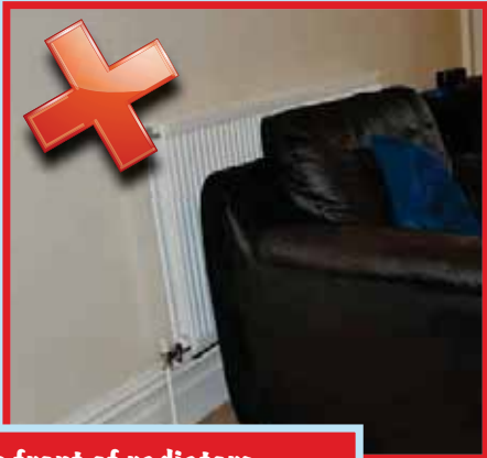
in front of radiators
